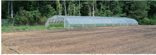
A hoop house was constructed in March to allow for year-round vegetable production.
